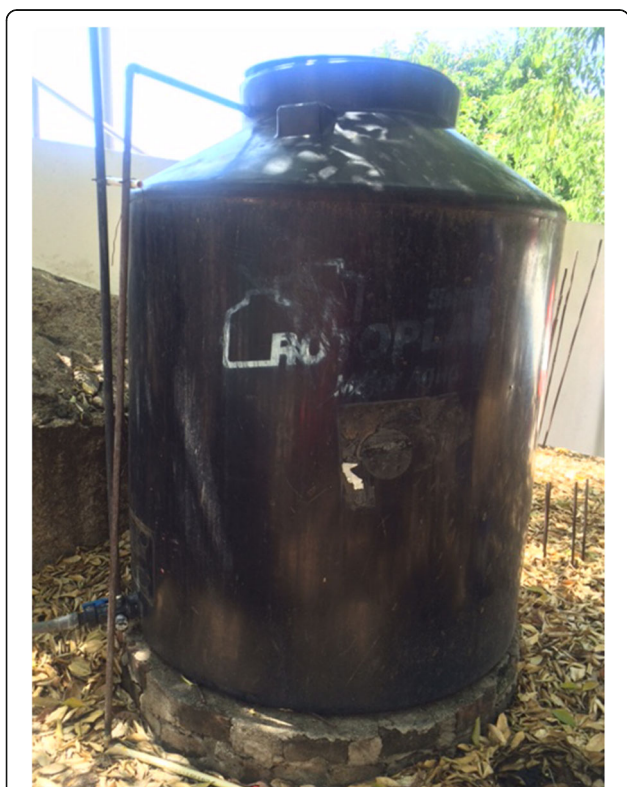
Fig. 4 A plastic water tank ( tinaco )
