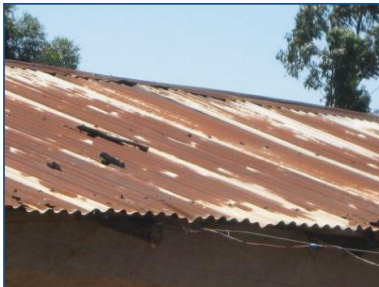
Figure 1 Corrosion on corrugated iron roof sheets close to factory due to air pollutions.
