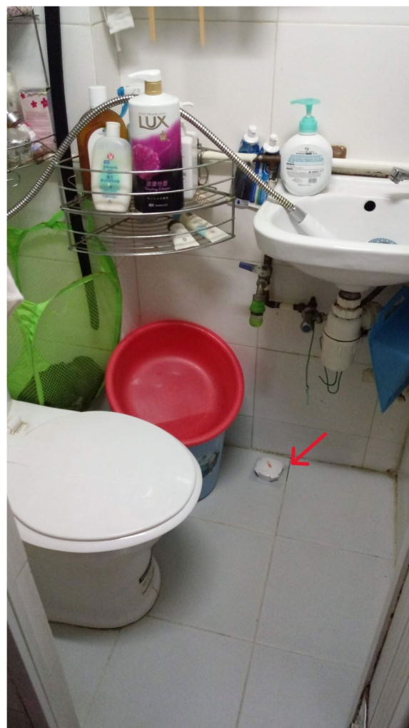
Fig. 7 The floor drain in Chan's bathroom was covered to avoid the backflow of wastewater
